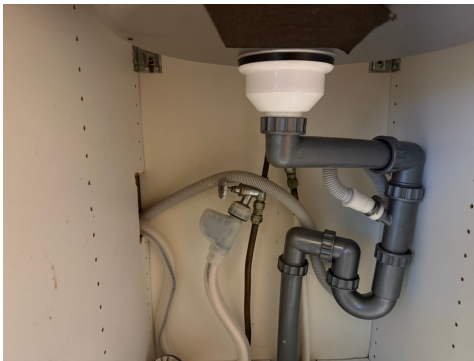
Røropplegg under vask.
